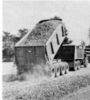
Laying a base course of crushed slag for the half million square foot parking lot, a Levy truck dumps the first half of its 20-ton legal load with a Gar Wood-St. Paul front-mounted telescopic hoist.
