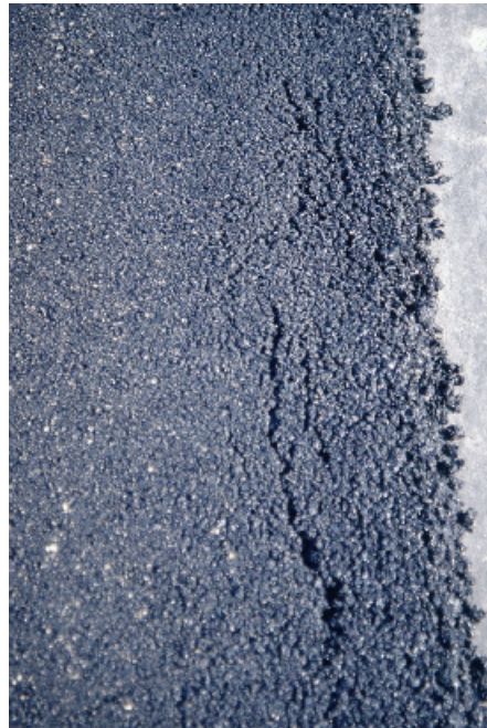
Figure 7. Crack formed at the edge of the lane due to the position of the edge of the roller drum
