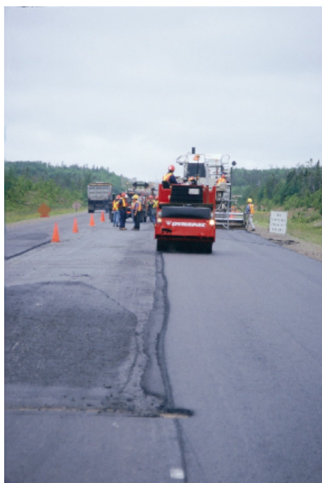
Figure 12. Transverse movement of the mix at the unsupported edge of pavement
