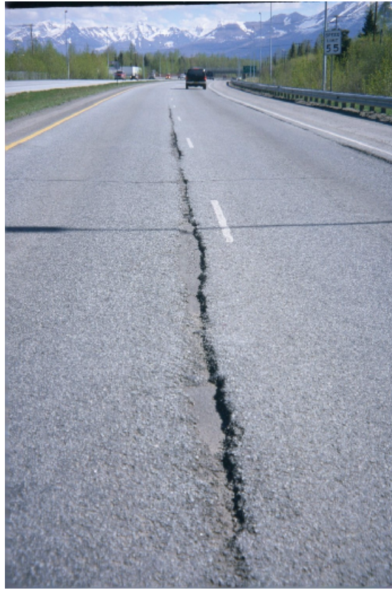
Figure 2. Severe erosion of mix at a longitudinal joint
