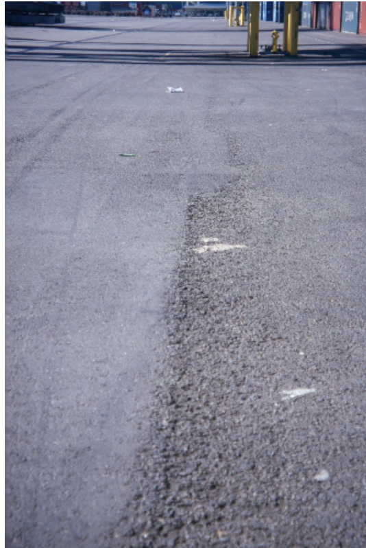
Figure 1. Raveling at a longitudinal joint
