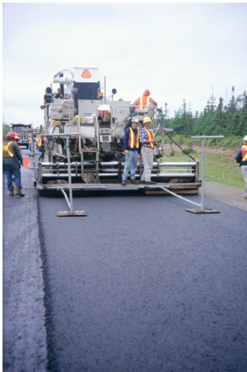
Figure 11. Paver placing unsupported edge of pavement
