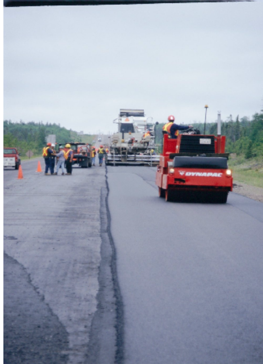
Figure 13. Transverse movement of the mix at the unsupported edge of pavement
