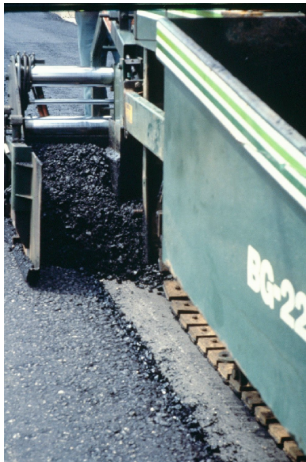
Figure 14. Excessive amount of overlap of mix from lane 2 over lane 1
