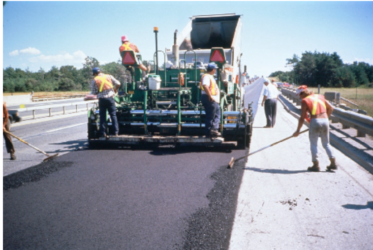
Figure 16. Improper raking of the longitudinal joint
