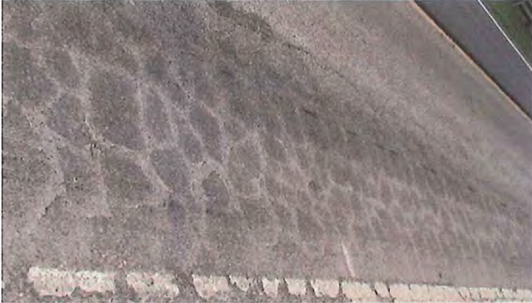
FIGURE 4 Pavement Distress Under Evotherm DAT Lift
