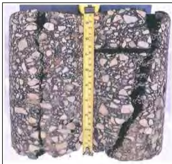
Figure 5.7: Core samples taken at transverse crack locations.
