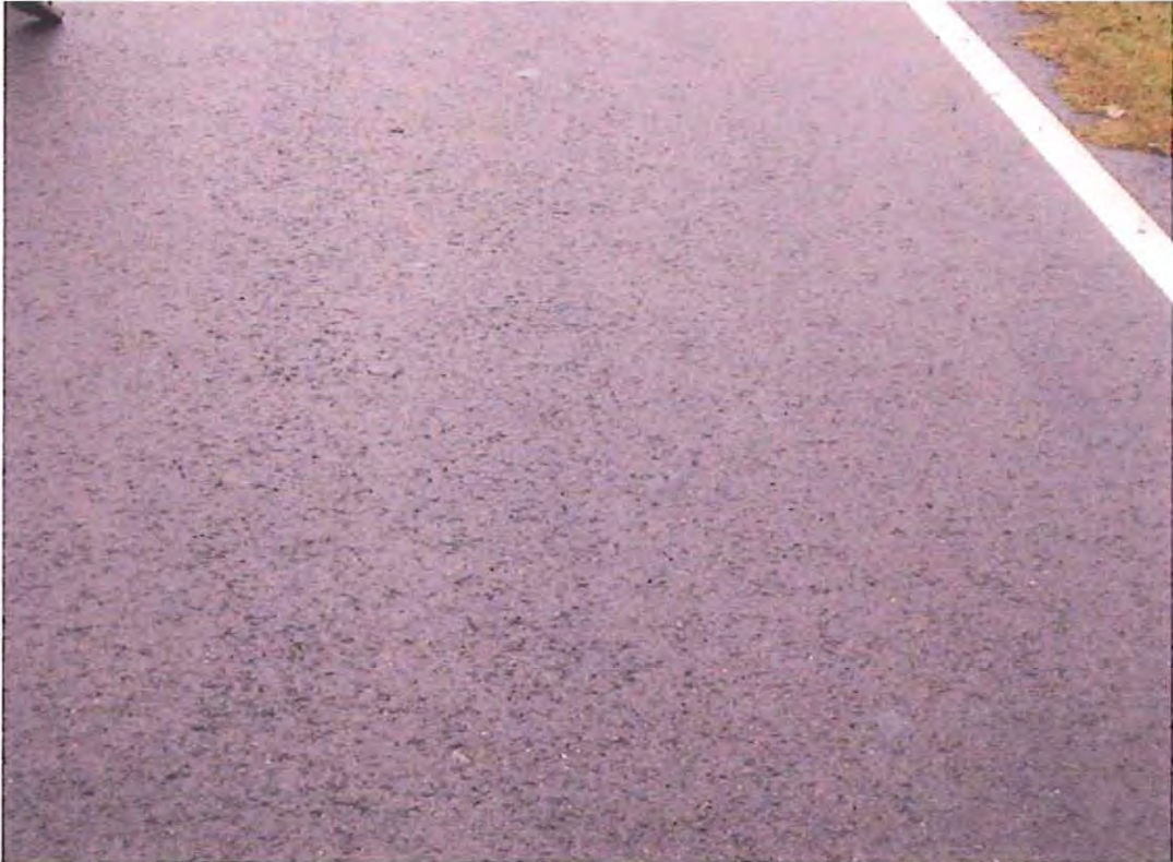
FIGURE 23 HMA 2 Pavement Condition
