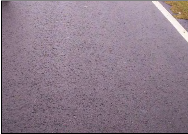
Figure 5.2: General view of the Control section.
