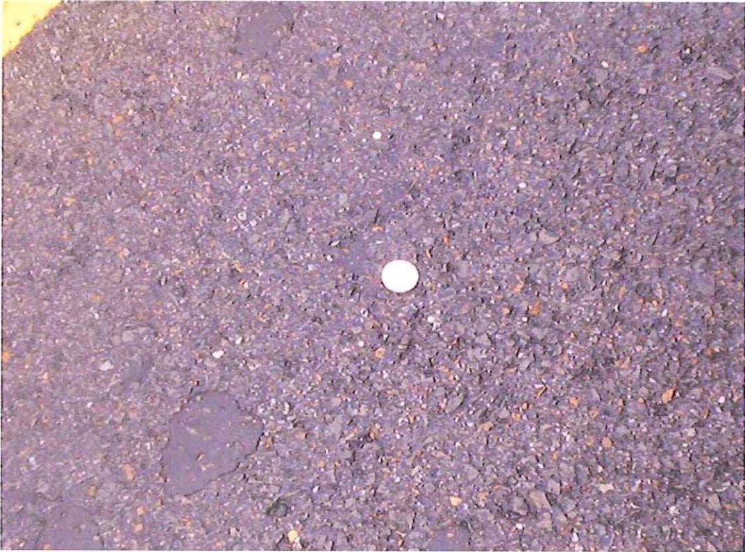
FIGURE 24 HMA 1 Pavement Condition
