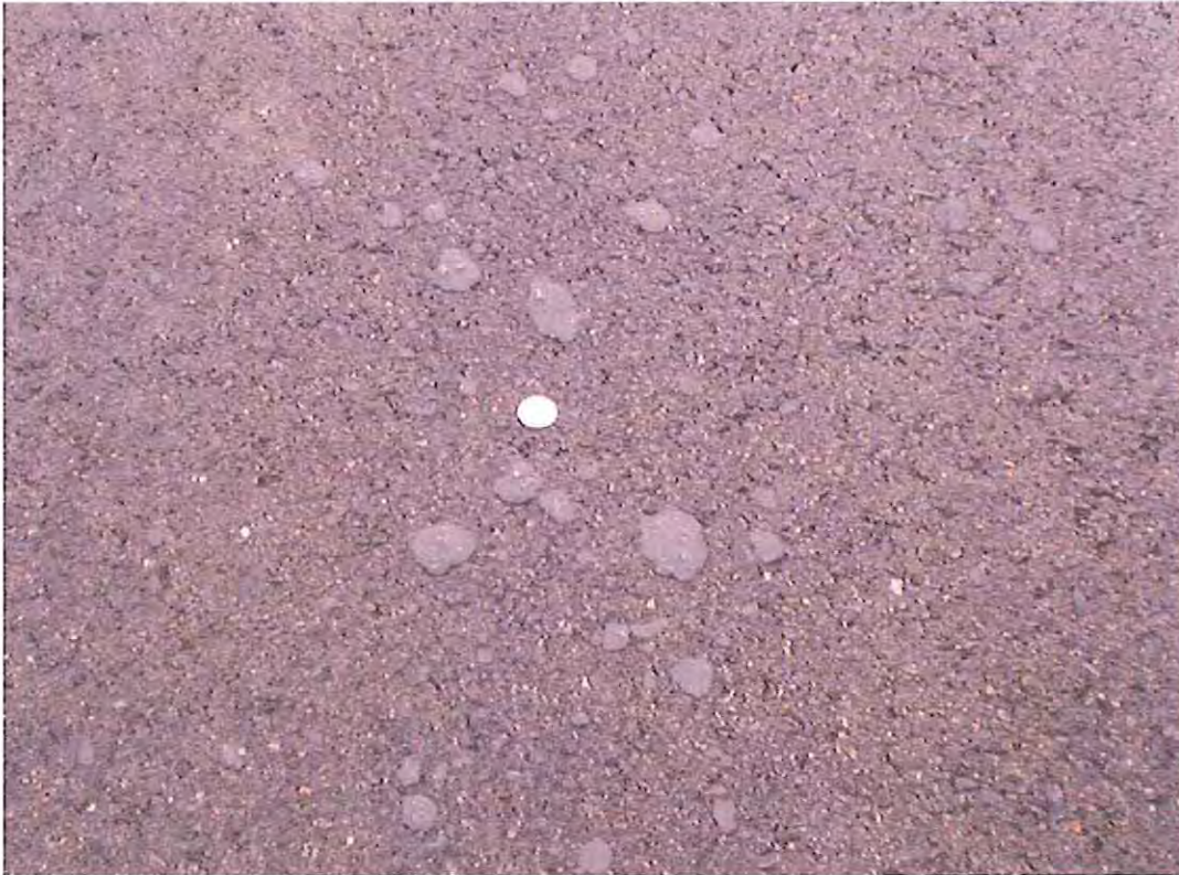
FIGURE 25 Advera Pavement Condition
