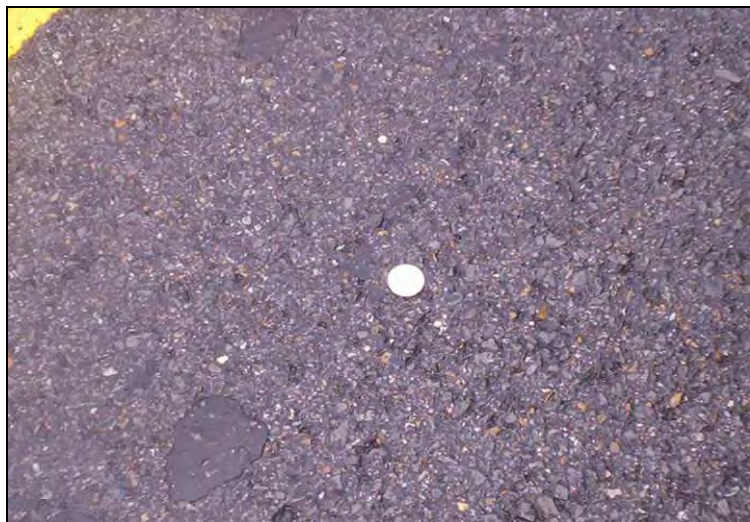
Figure 5.3: Close-up view of the Control section.
