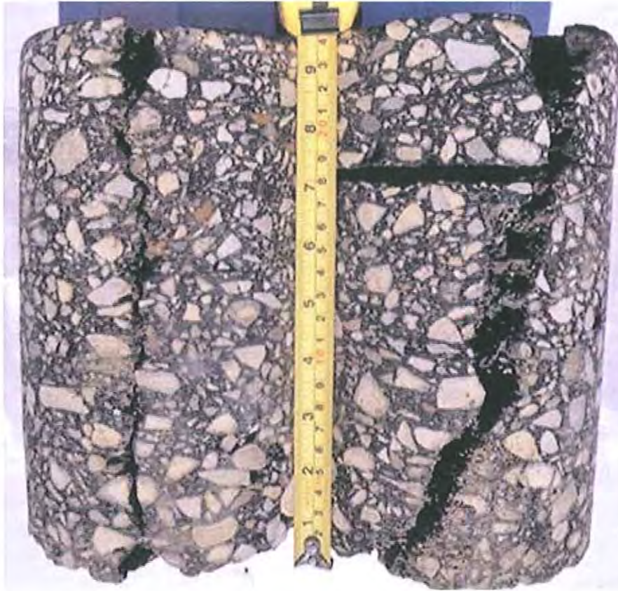
Figure 9. Core Samples Taken at Transverse Crack Locations
