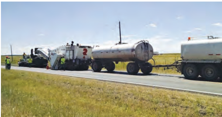
Cold In-Place Recycling Single Unit Train with Water Truck, Emulsion Tanker, Milling machine and Paver in Arapahoe County
