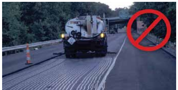
Figure 5-3. Non-Uniform Tack Coat Spray Application With Blocked and Oversize Nozzles
