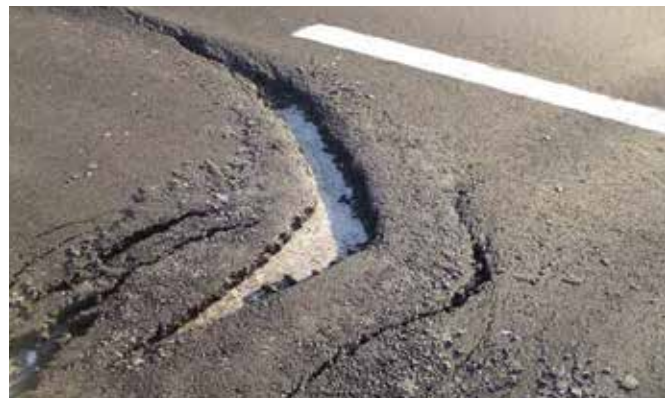
Figure 4-1. Delamination Type of Sliding Failure
