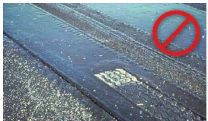
Figure 5-6. Excessive Tack Coat Spray Application
