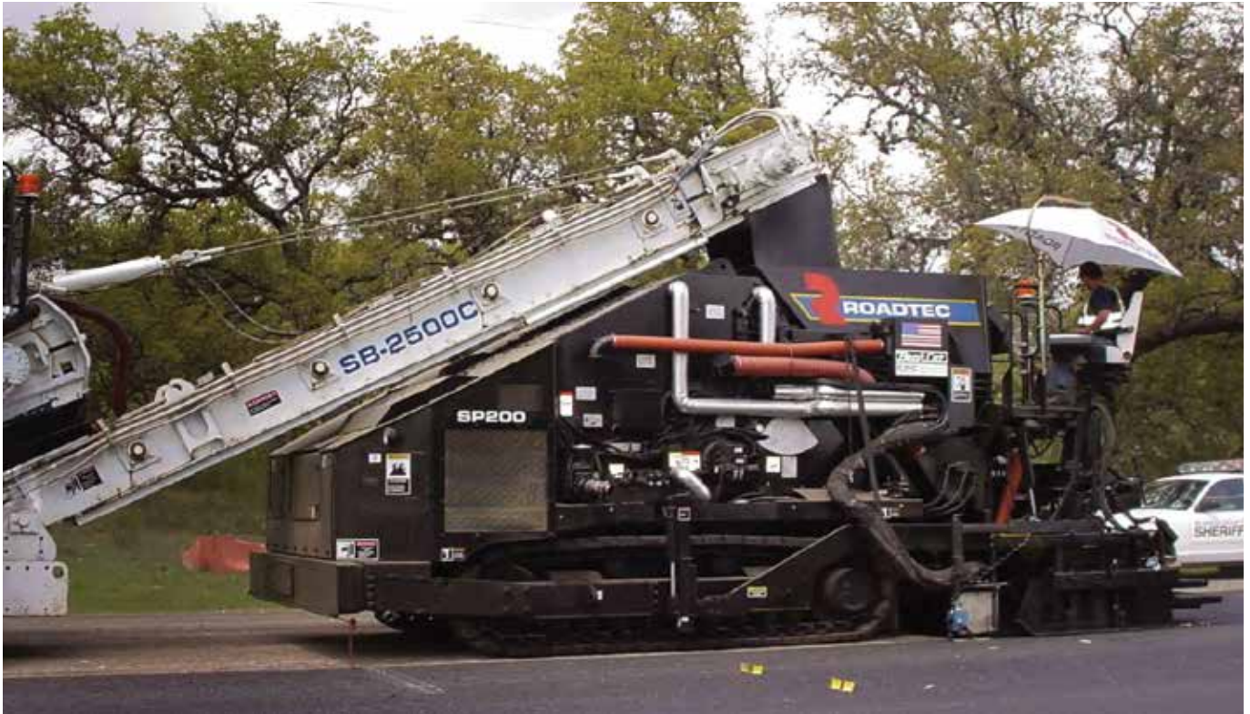
Figures 3-17. Spray Paver With the Spray Bar Located Between Track and Screed
