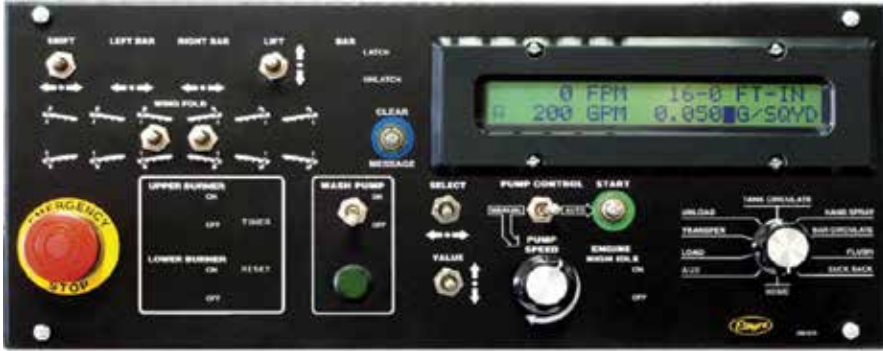
Figure 3-3. Control Panel in Distributor Truck
