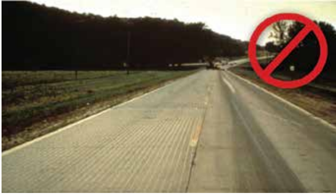
Figure 3-8. Poor Spray Pattern of Tack Coat Due to Improper Nozzle Alignment, Nozzle Size, and/or Pump Pressure
