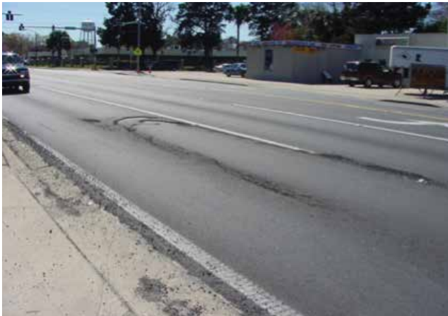
Figure 1. Slippage Cracking (FDOT)
