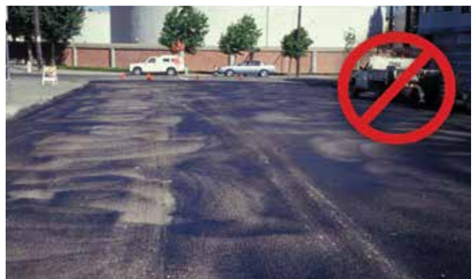
Figure 3-14. Improper Application of the Tack Coat Using a Hand Wand
