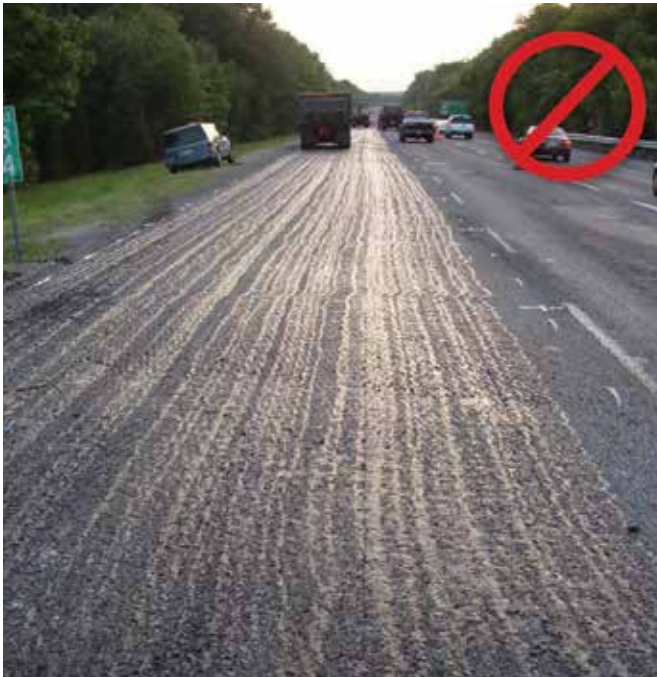
Figure 5-7. Non-Uniform Tack Coat Spray Application With Nozzles Not Functioning and Not at the Correct Angle
