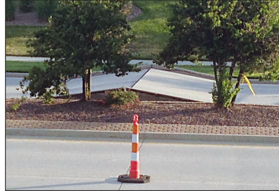
Buckeled concrete panels in Arapahoe County
