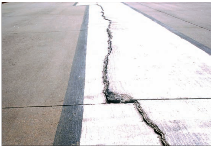
Distressed concrete pavement at the Yuma Municipal Airport
