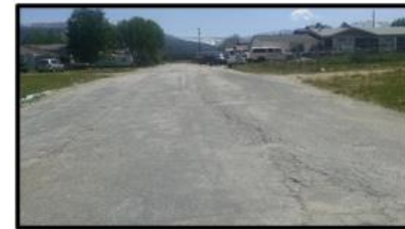
'Poor' Condition (PCI < 41)
